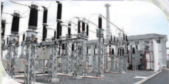
Substation 10/22kv 110/22KV
